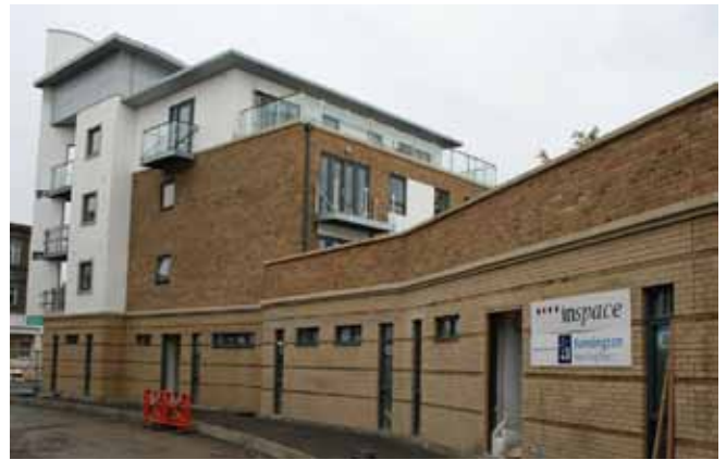
Building work nears completion on 12 ground-floor studios at Harrow Road, NW10. Photo: Acme Studios (2009)
